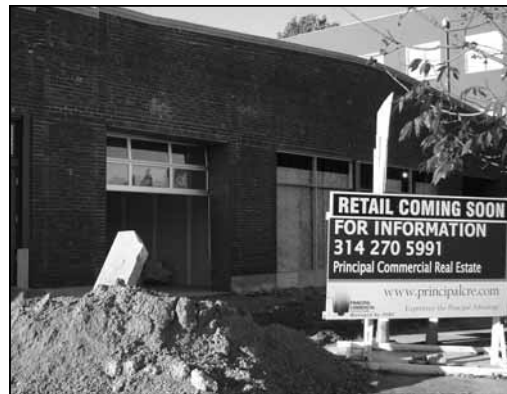
The rehab continues at Neal Shapiro's former Original Cast Lighting Building next to the Regional Arts Commission on Delmar. The first tenant will be a new Italian restaurant from the Del Pietro family, set to open later this month.
