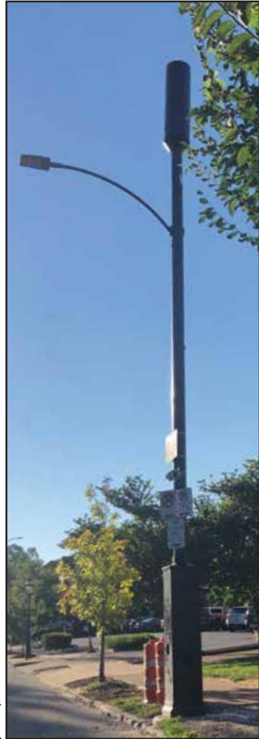
New 5G light pole at 4400 Maryland
